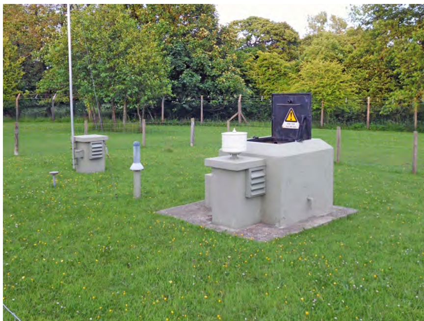
The surface features in their third reincarnation in Goosnargh, with vents, hatch, GZI, FSM probe head and BPI baffle all in position in 2013. Catforth post never had a radio, so currently this is only a representative item. Photo Mike Norris
